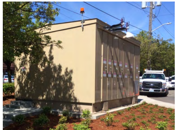
Typical TPSS (located at Broadway and Minor Ave)
